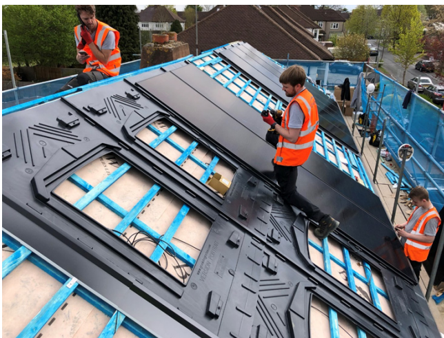
Baily Garner is providing full PAS 2035 services and retrofit expertise on Raven Housing Trust's SHDF Wave 2.1 project after successfully assisting in the completion of its Wave 1 scheme
